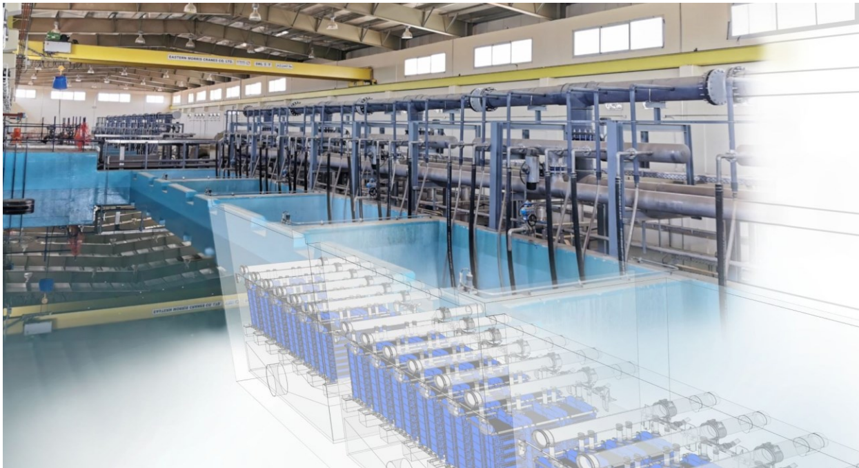
CERAFILTEC project. In operation Q4 2021
