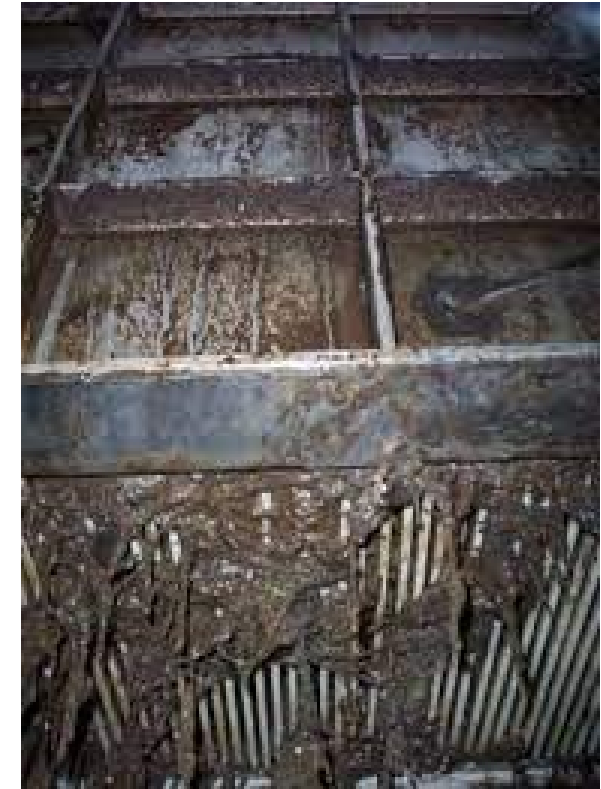
Plastic membranes after heavy use. Fully clogged. Fiber breaking
